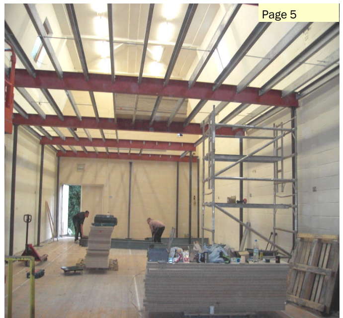
Conversion of the lodge to provide 7 new offices and EQ therapy hall
